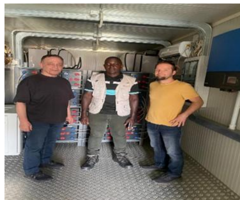
Figure 12: Inside The Power House with the Mini grid operator
