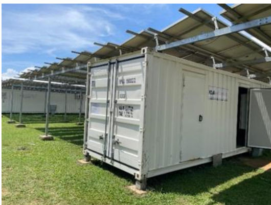
Figure 11: The 8KWp Mini grid by Winch Energy on Bunjako Island
